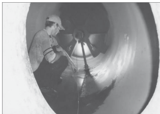
Fig. 27 Interior of cylinder without condensate, after reconstruction
